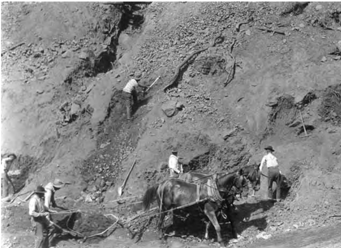
A two-horse drawn Fresno Scraper at work building the Magalia Dam sometime after 1916. The man in the foreground is driving the team while the man next to him uses a loop-shaped lever to tilt the scraper blade into the ground. This was state-of-the-art in those days. Paradise Irrigation District.
