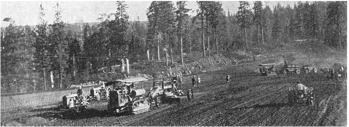
A photo of the construction site showing some of the many pieces of equipment on the job. Western Construction News.
